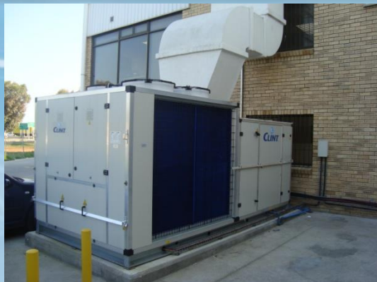
SOUTH AFRICA JOHANNESBURG UWC Metrology Lab
